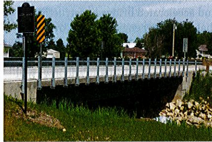
The Jesup South Bridge served as a demonstration project to affirm the value of the eSPAN140 tool for bridge design.
