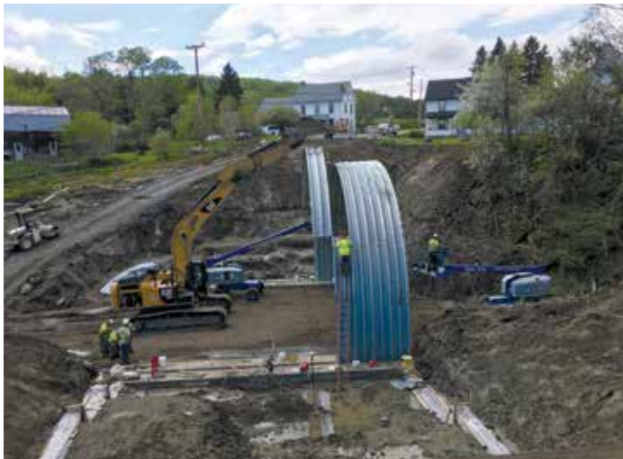
Figure 2. Plates being assembled on the Route 2B Bridge replacement project in St. Johnsbury, Vermont.
