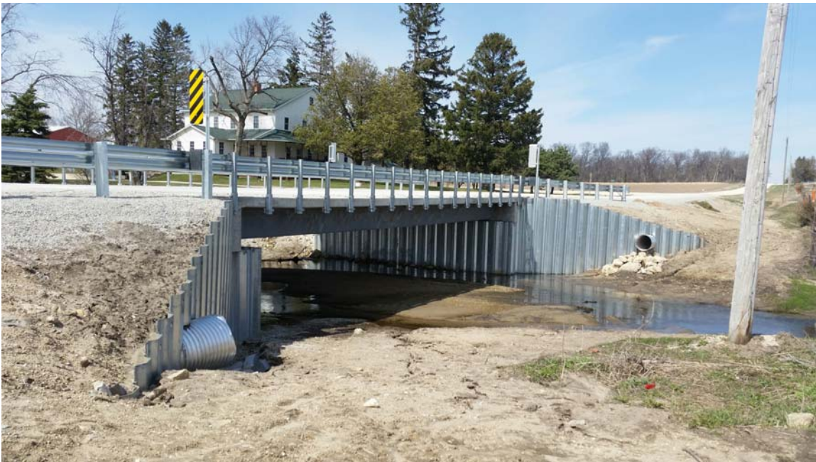
The new Amish Sawmill Bridge is the first press-brake-formed steel tub girder bridge constructed in the United States. Additional projects are in the planning stages in Ohio and West Virginia.
