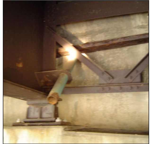
Broken pipe of drainage system pictured.
