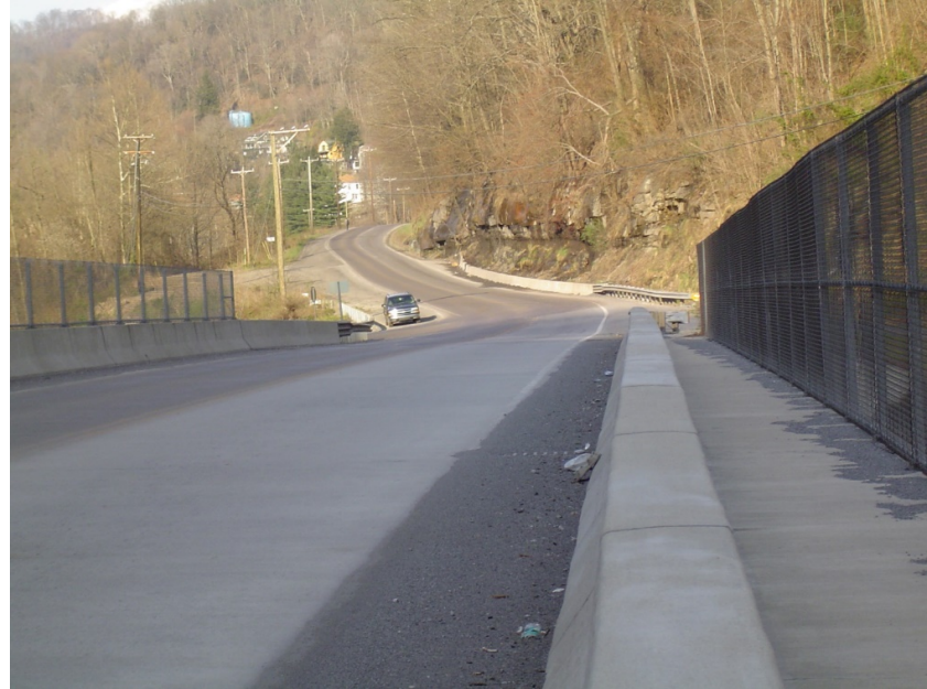
Blocked scuppers pictured.
